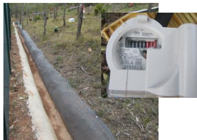
Trenches and water counters
